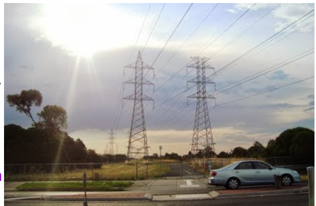
Illustration 1: Electricity transmission towers at Glenroy during Heatwave
